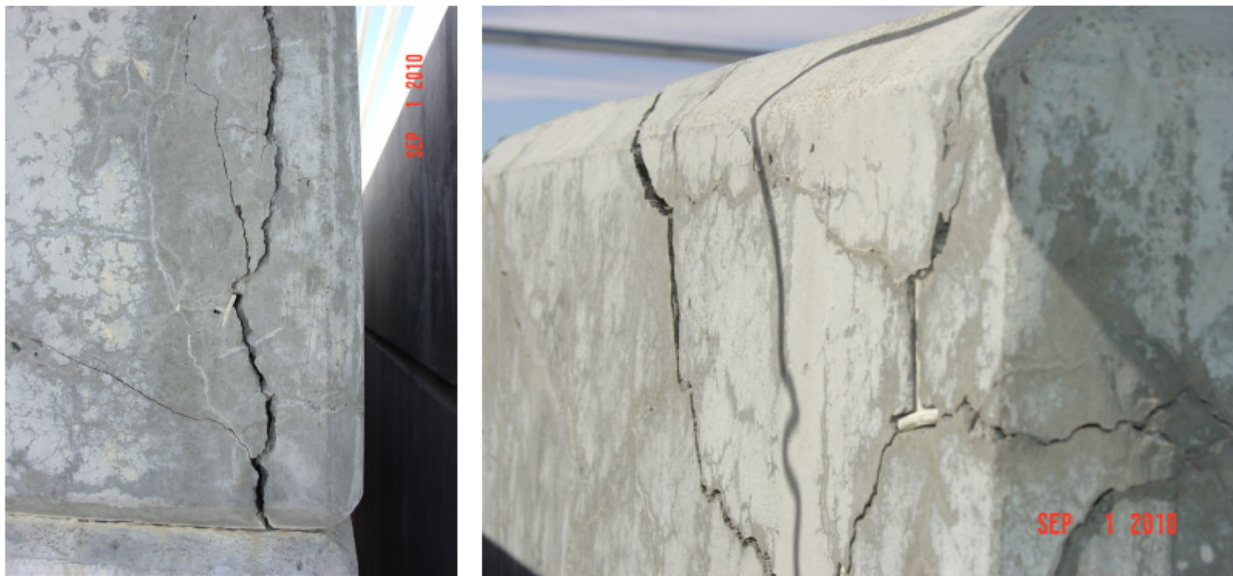
Figure 1 Two examples from north west (left) and north east (right) corner roof damage of a horizontal storage module at the site of Three Mile Island Unit 2 (NRC 2012)
