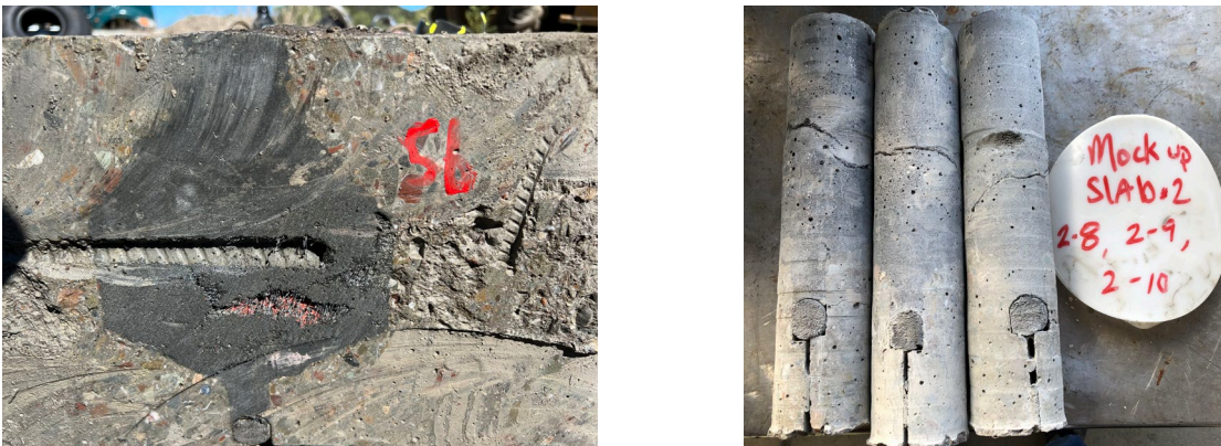
Figure 1. Voids and Cold Joints Observed After Saw Cutting and Coring Mockups.
